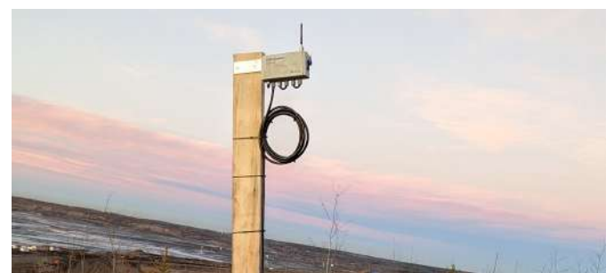
Five-channel vibrating-wire node installed on wooden post.
