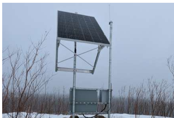
Solar powered Gateway installation designed for two weeks of autonomy.
