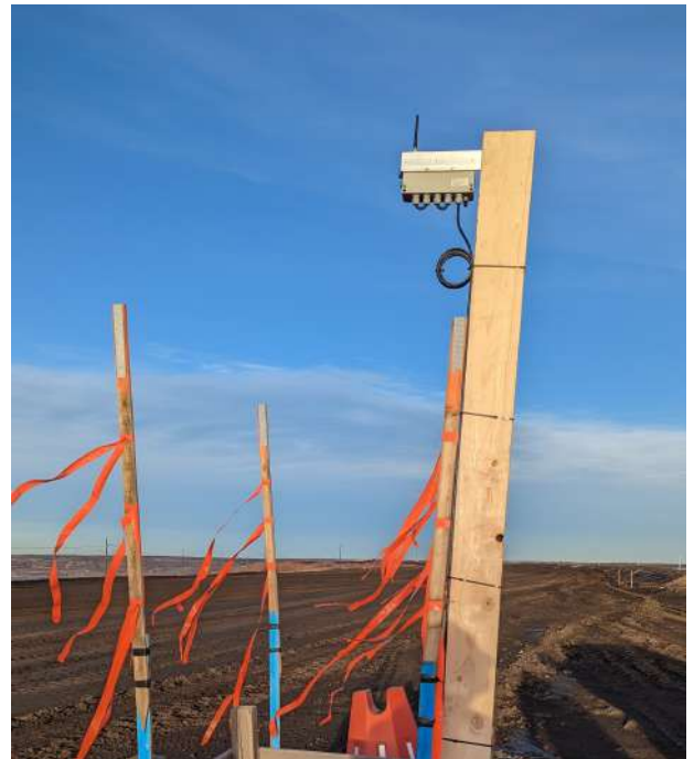
Five-channel vibrating-wire node installed on wooden post.
