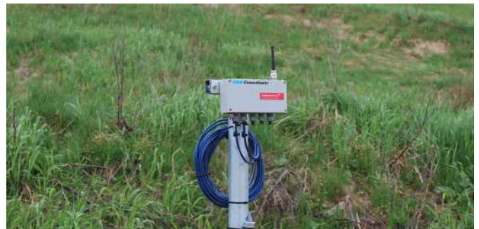
Five channel vibrating wire node installed on post
