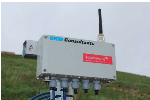
Five channel vibrating wire node installed on post, ready for dike raise
