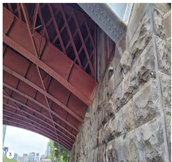
Figures 3: Tiltmeters installed under a bridge.
