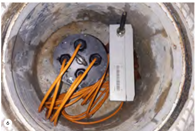
Figures 4, 5 and 6: Gateway gathering data from tiltmeters and extensometers installed with data loggers on the track.
