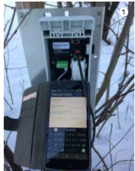
1 - Loadsensing data node being configured simply through a mobile application
