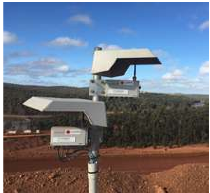
WorldSensing Vibrating Wire 5-channel data logger installation
